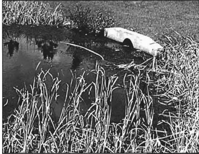
▲ Typical inflow pipe.
